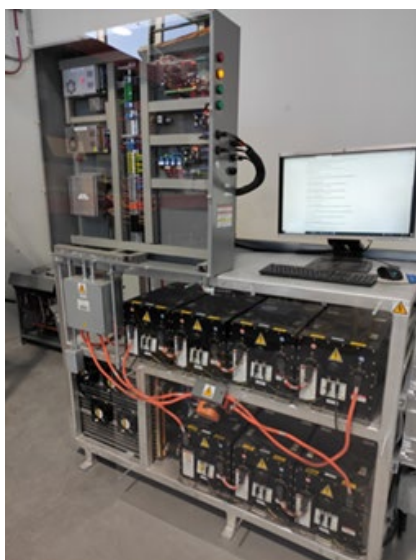
Figure 5 – Battery rack inside
