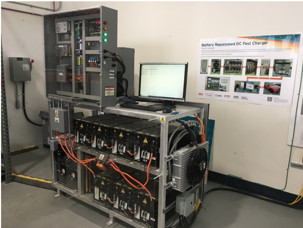
Figure 2. Battery energy storage system (BESS) set-up inside CARSI Building for the B2U at RRC Polytech, Notre Dame Campus, Winnipeg (R. Parsons 2022).
