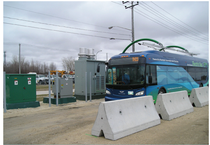
Figure 3: Manitoba Hydro Rapid Charger Station Installation for Phase 3
