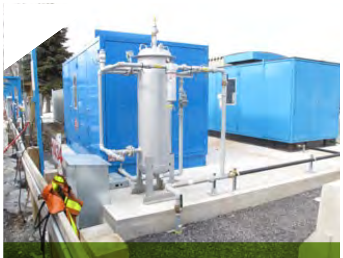
Figure 12 - Sulzer Compressor Station
