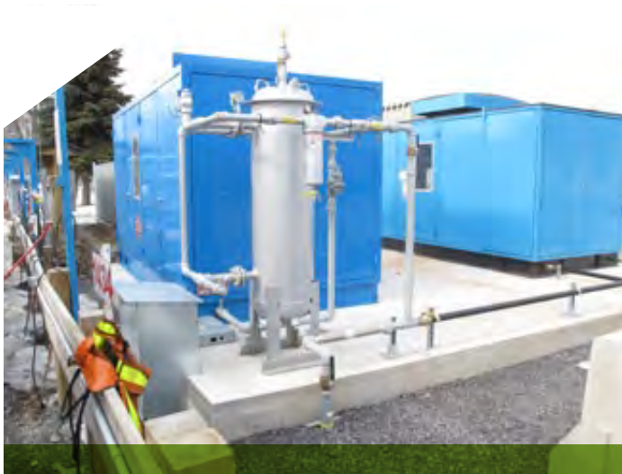
Figure 13 - PSB Natural Gas Dryer
