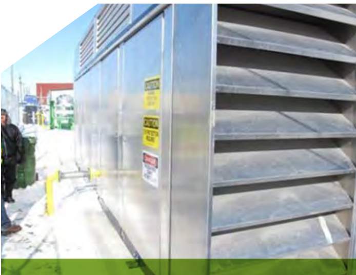
Figure 29 - Compressor Station Enclosure
