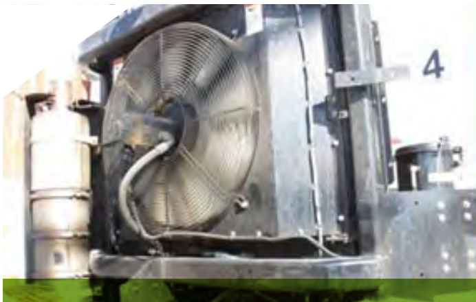
Figure 25 - Behind Cab Radiator Cooling System
