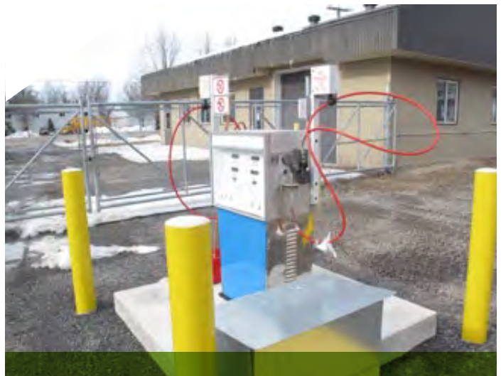
Figure 17 - Fast Fill Dispenser
