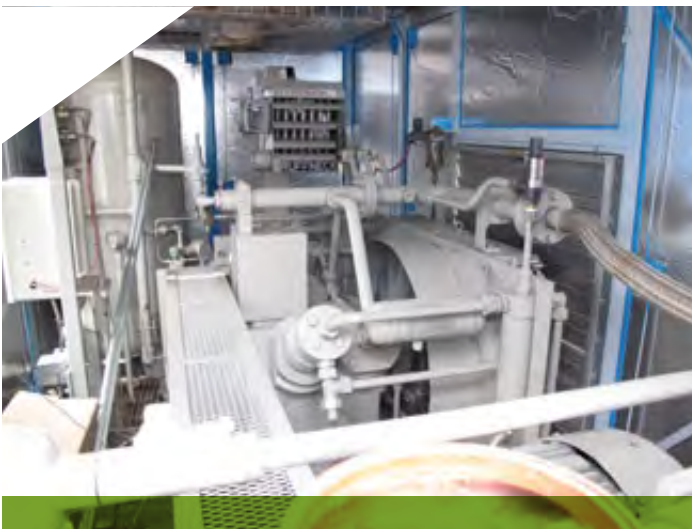
Figure 16 - Equipment Inside Station Enclosure
