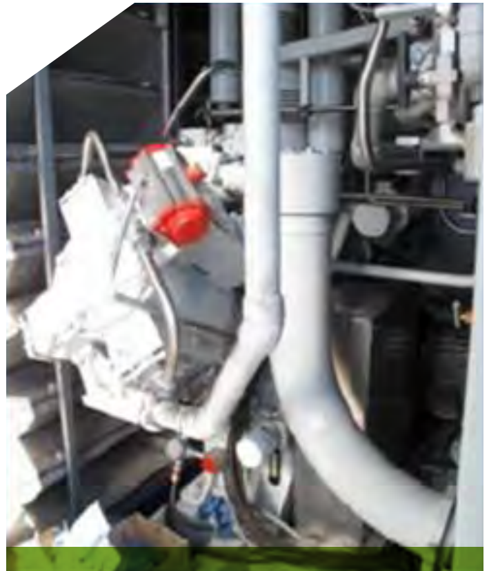
Figure 30 - Equipment Inside Enclosure
