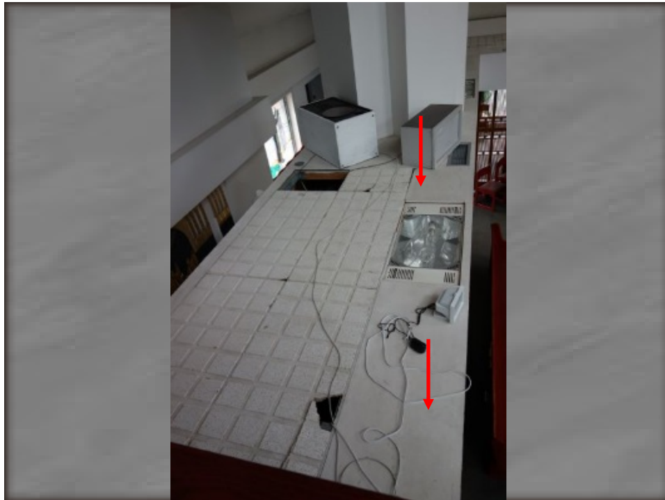
Figure 11 – Top of Perimeter Ring Open to Interior Space (NOTE: Openings as found indicated by red arrows)
