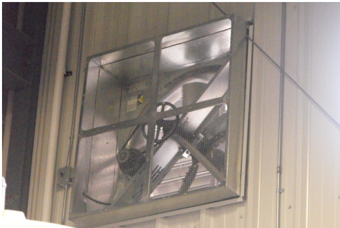
Figure 5 – Exhaust Fan with Backdraft Dampers
